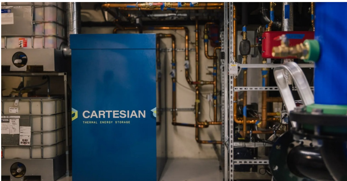
The Cartesian Thermal Box beside the CO 2 heat pump in the plant room. A thermal water tank would have been about eight times larger. Photo: Martin Håndlykken.
